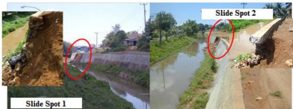
Figure 2. The condition of barrier slide (Slide 1, Sta. 0+650) and (Slide 2, Sta. 0+950)
