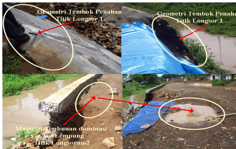
Figure 6. The construction material for pavement and protection wall at both slide spots.
