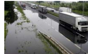
Inundation due to ill-dimensioned drainage systems
