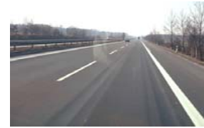
Increase in rutting
