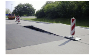
More "Blow ups" in concrete surfaces
